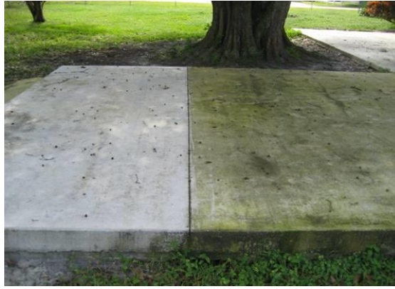
Figure 4: Images of existing concrete slabs: DCE-treated (left) and untreated (right). No cleaning was made to the surface prior to applying the DCE.
